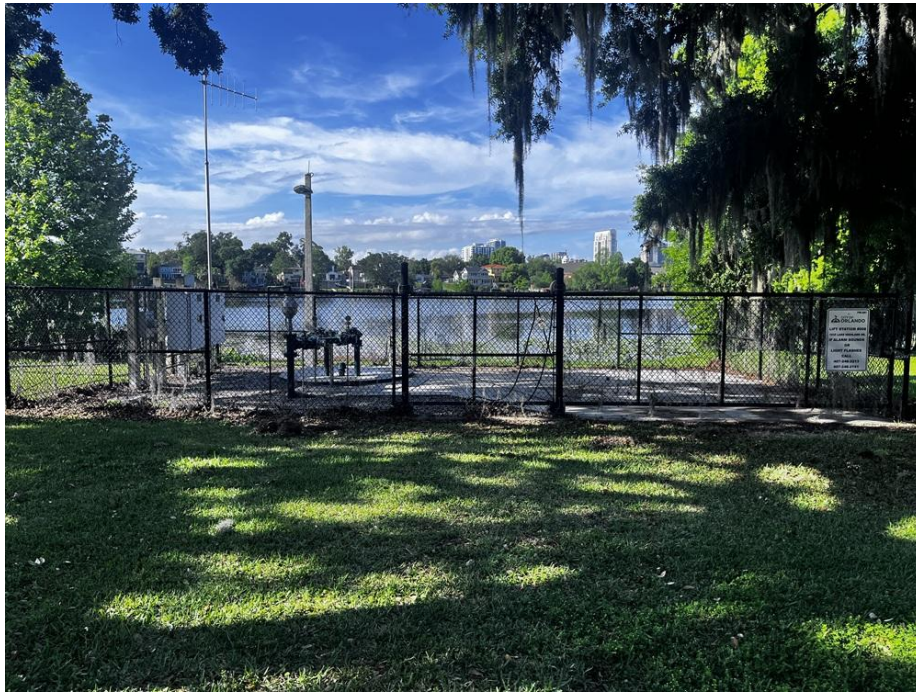
View south of lift station at Lake Highland
