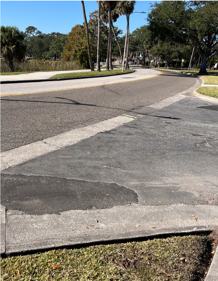
5 Deterioration of site or other improvements.
