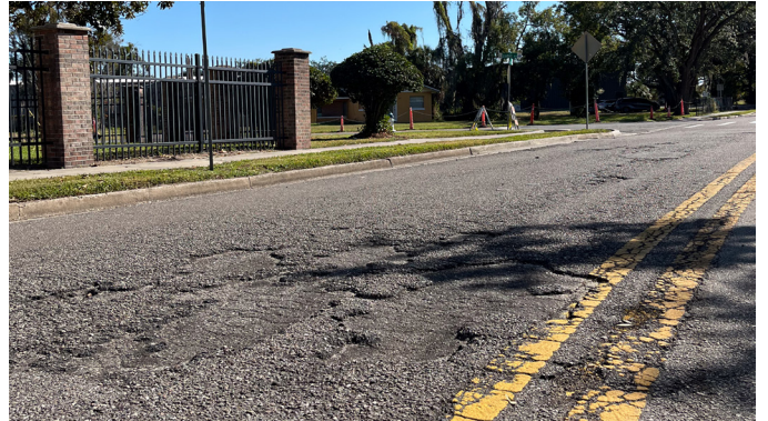
6 Deterioration of site or other improvements.
